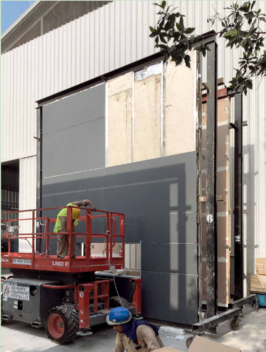
Setting up for an on-site fire safety test.
